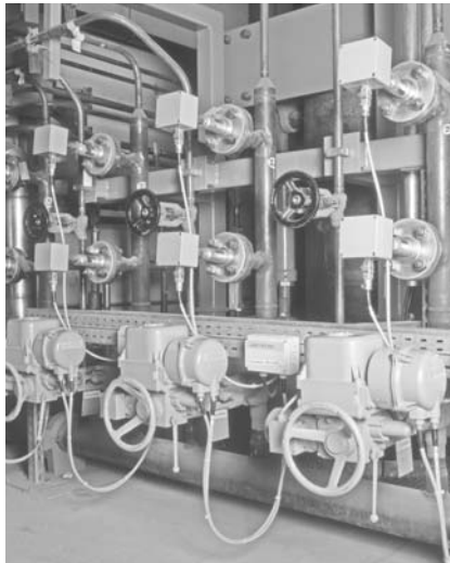
Drain control station using ZK 29 valves with electrical actuator
